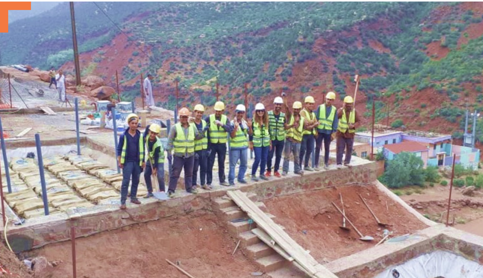
Salma Bougarrani and her colleagues at the construction site of Green WATECH wastewater treatment plant in the Igri village, High Atlas Mountains in Morocco
